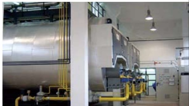
Szczecin and Konin Power Plant
